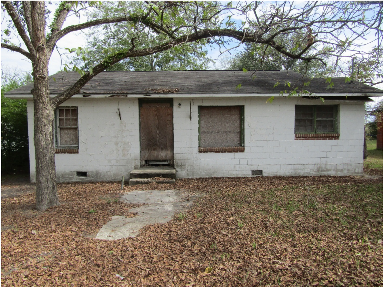
Figure 40: Substandard single-family home located on Thomas Street.
