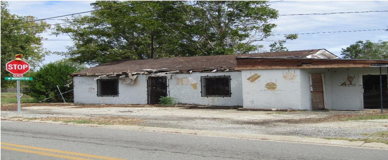
Figure 38: Substandard building on Thomas Street at the T junction of Bennett Street
