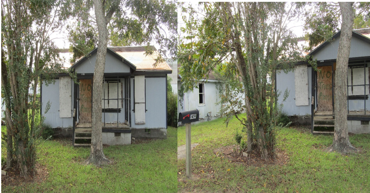
Figure 36: Substandard vacant building on Beacon Street
