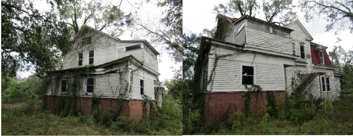
Figure 29: Property on North Peachtree Street beside a Multi-family units 245 N Peachtree Street. Building is severely damaged.
