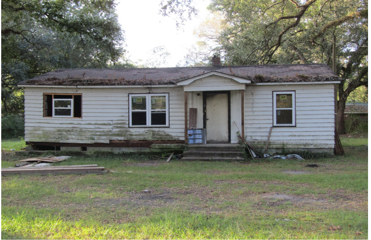
Figure 42: Substandard single-family home located on McRee Street.
