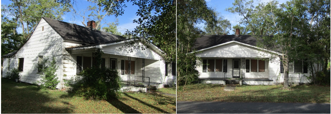
Figure 41: Substandard single-family home located on Thomas Street.
